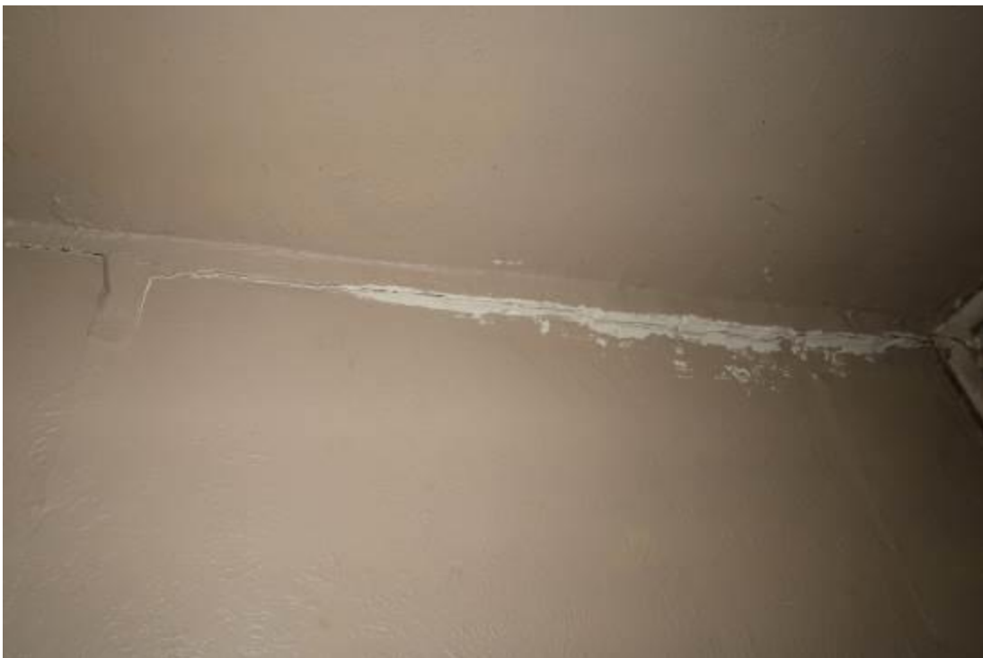
Wall Damage (Inverted Photograph)
