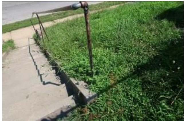
Damaged Safety Railing
