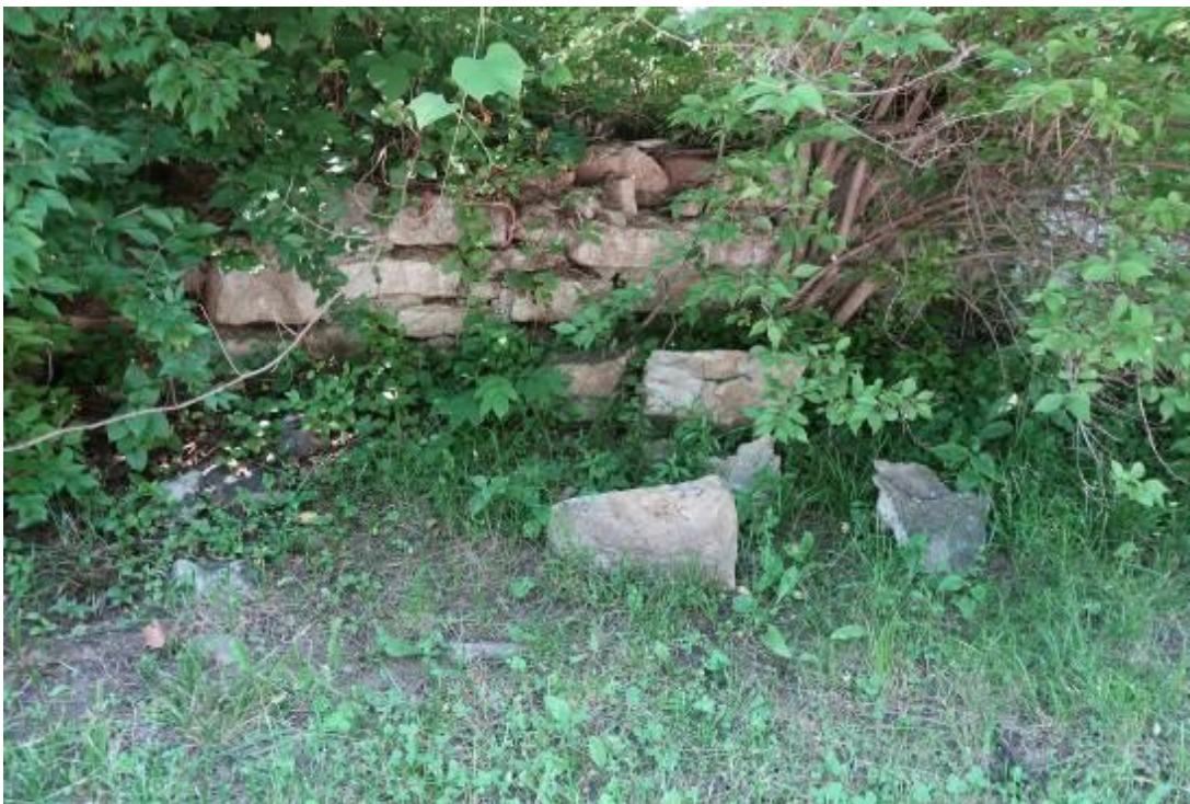
Collapsing Retaining Wall Along E 62 nd Street
