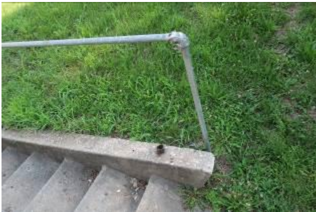
Damaged Safety Railing
