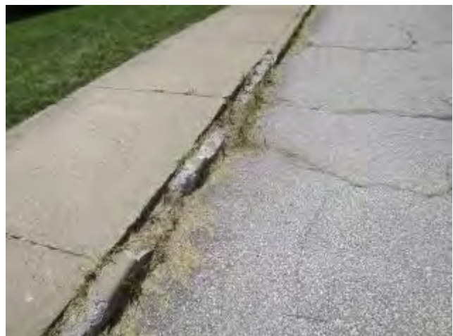
Deteriorated Curbs At 2801 Swope Parkway
