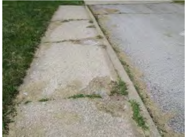
Deteriorating Sidewalk At 2801 Swope Parkway
