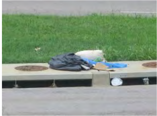
Trash At Sewer Inlet On Swope Parkway
