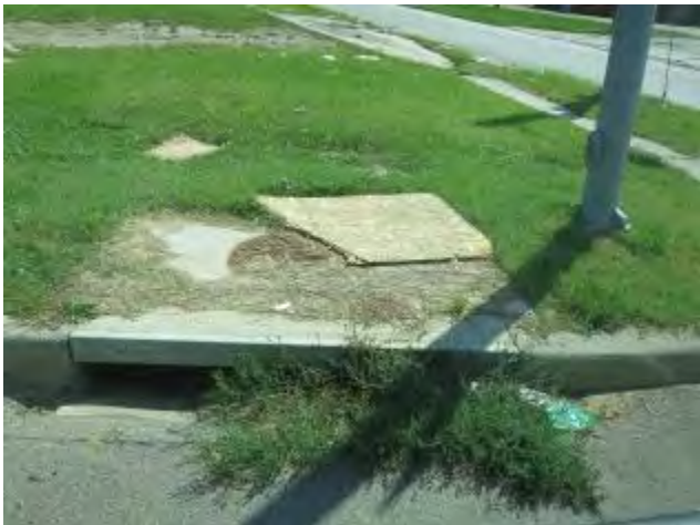
Clogged Sewer Inlet Along Swope Parkway
