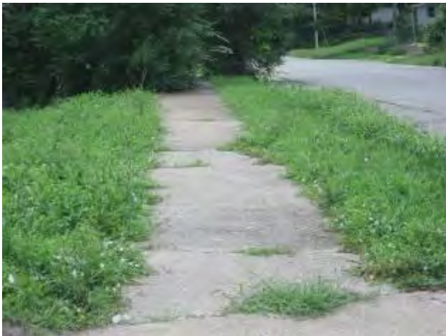
Deteriorating Sidewalk Along Agnes Avenue
