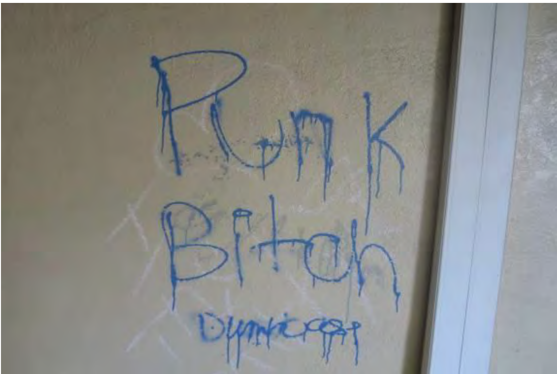
Trespassing/Vandalism/Graffiti At 2801 Swope Parkway
