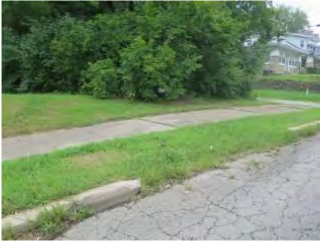
Deteriorating Curbs & Lack Of Gutters – College Ave.
