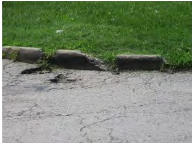
Deteriorated Curbs Along Agnes Avenue
