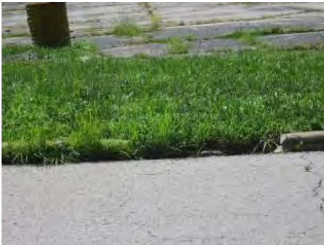
Deteriorated Curbs Along Agnes Avenue
