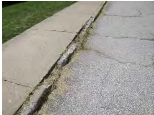
Deteriorated Curbs At 2801 Swope Parkway
