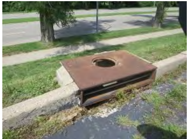
Deteriorating Sewer Inlet At 3011 Swope Parkway
