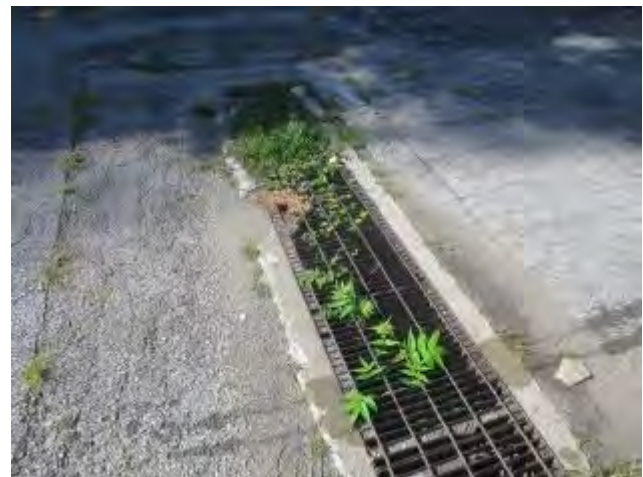
Clogged Drainage Grate At 2915 Swope Parkway
