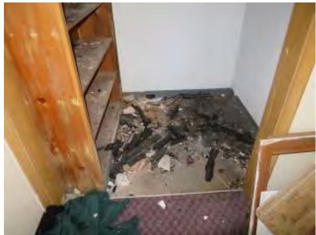
Interior Fire At 2801 Swope Parkway
