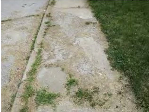
Deteriorating Sidewalk At 2801 Swope Parkway
