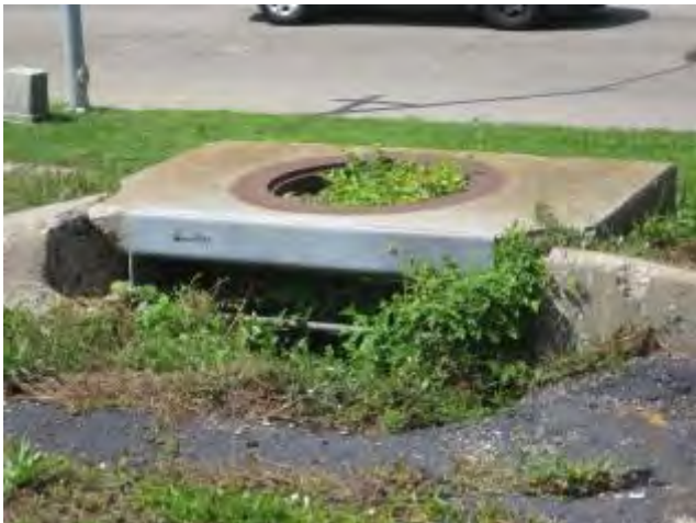
Clogged Sewer Inlet At 3011 Swope Parkway
