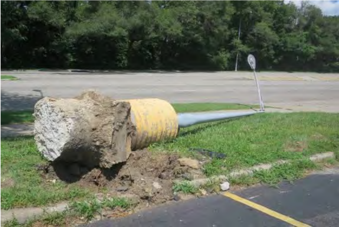
Collapsed Parking Lot Lamppost – 3011 Swope Parkway
