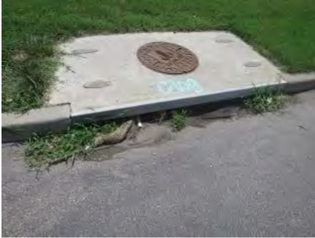
Clogged Sewer Inlet Along Swope Parkway
