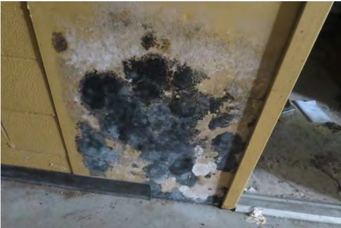
Water Infiltration And Black Mold – 2801 Swope Parkway
