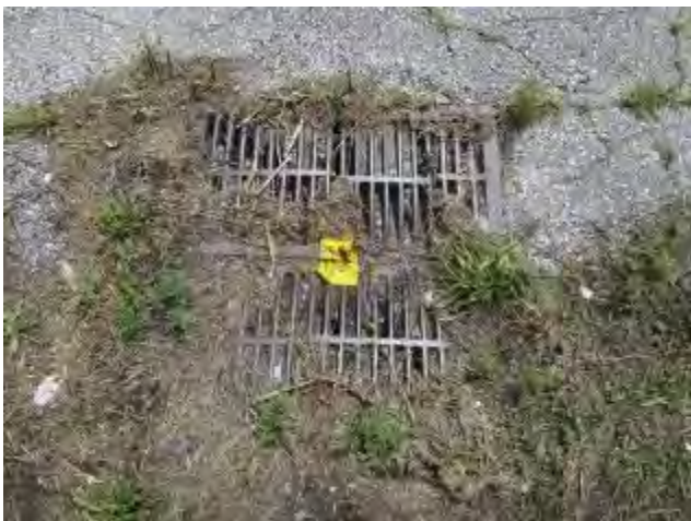
Clogged Sewer Inlet At 2801 Swope Parkway
