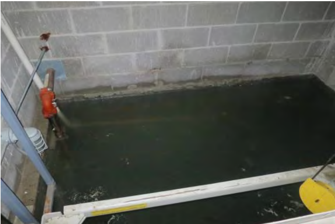
Water-Filled Elevator Shaft – 2801 Swope Parkway
