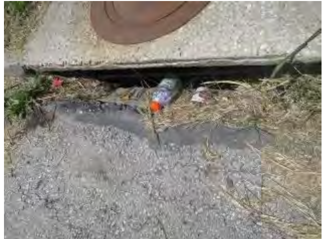
Clogged Sewer Inlet Along E 49th Street
