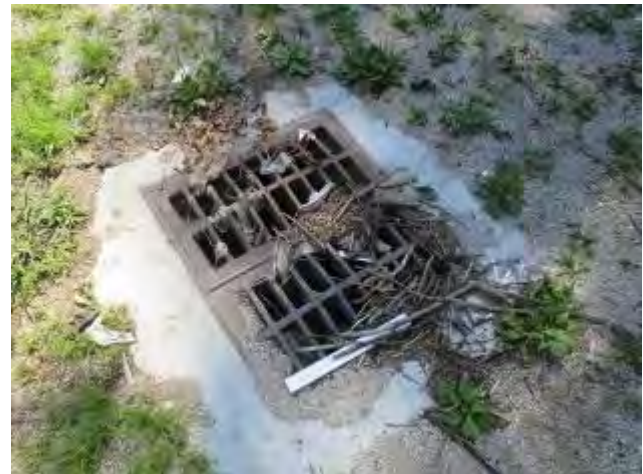
Clogged Sewer Inlet At 3011 Swope Parkway
