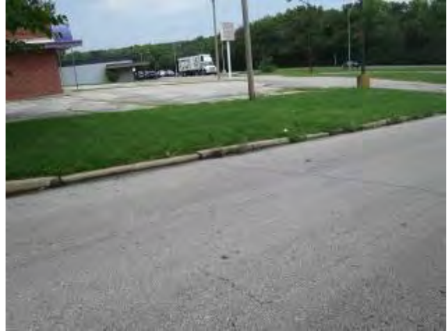
Deteriorating Curbs Along College Avenue
