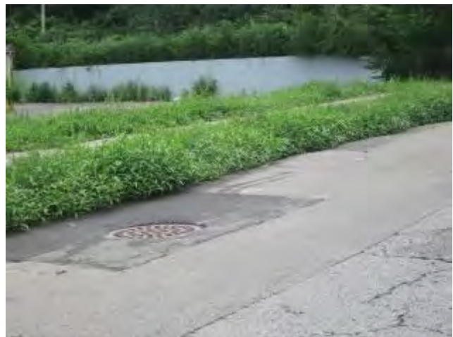
Lack Of Curbs & Gutters Along Agnes Avenue
