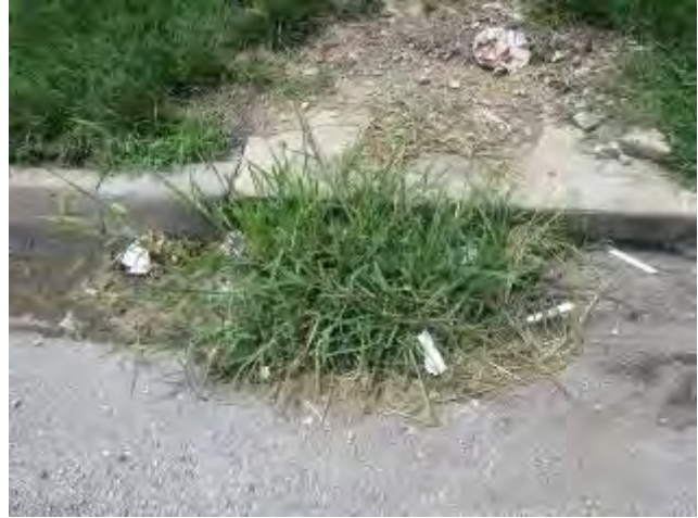
Clogged Sewer Inlet Along Chestnut Avenue
