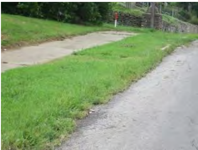
Lack Of Curbs & Gutters Along College Avenue
