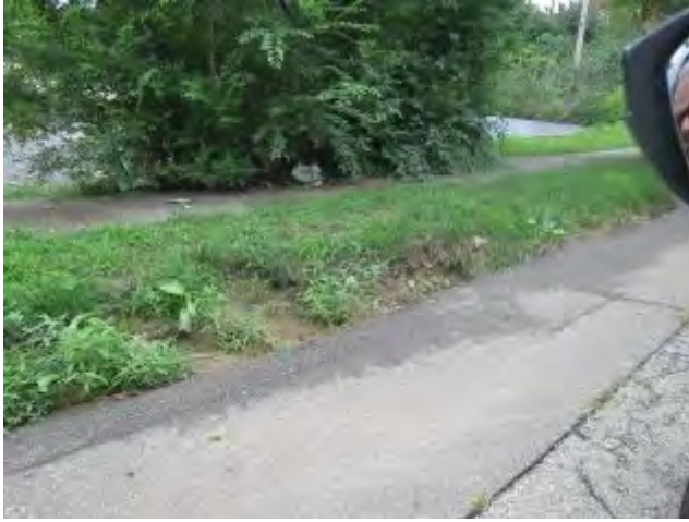
Lack Of Curbs & Gutters Along Agnes Avenue
