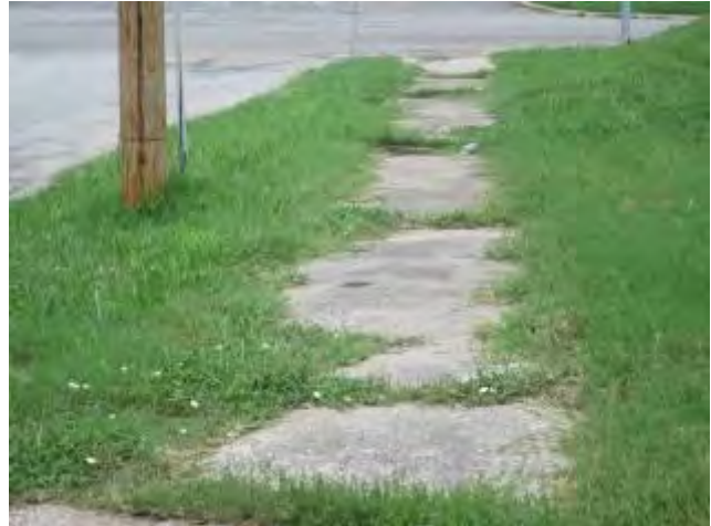
Deteriorating/Unsafe Sidewalk Along Agnes Avenue
