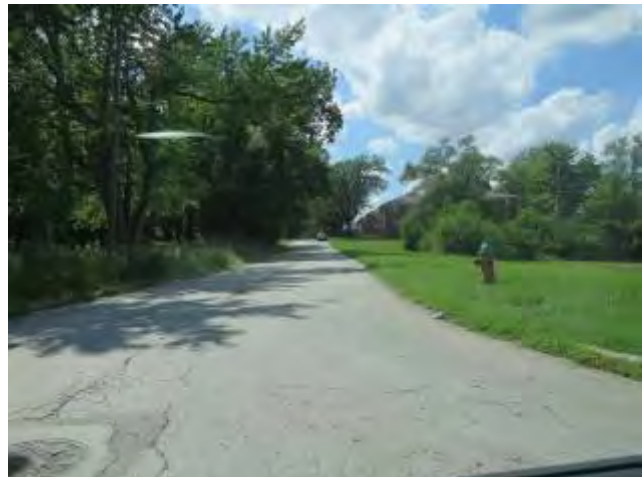
Lack Of Curbs & Gutters Along E 49th Street
