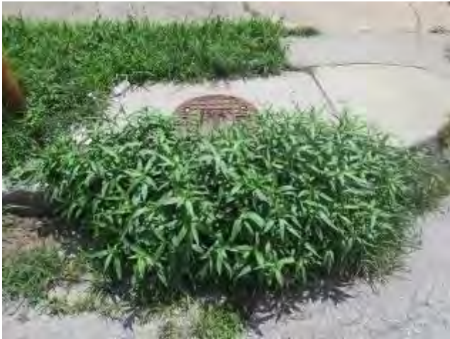
Clogged Sewer Inlet Along E 49th Street
