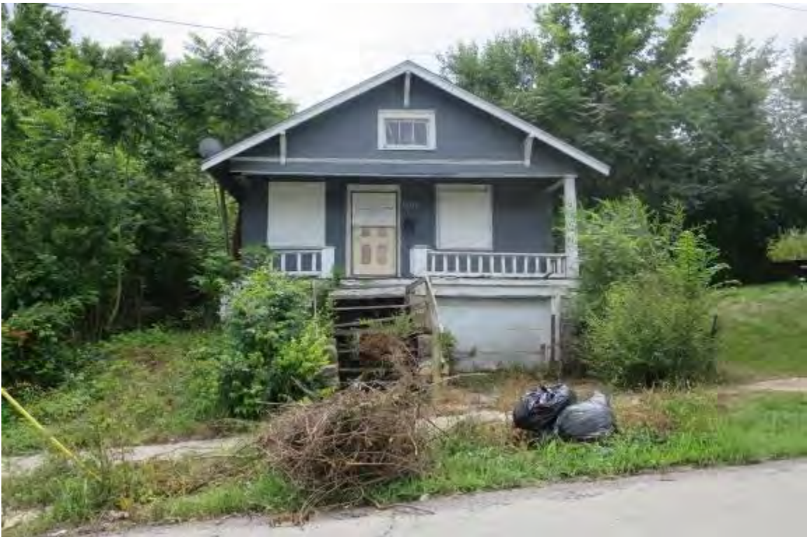
Dangerous Building Citation (2709 E 49 th Street) – Southeast Of Study Area
