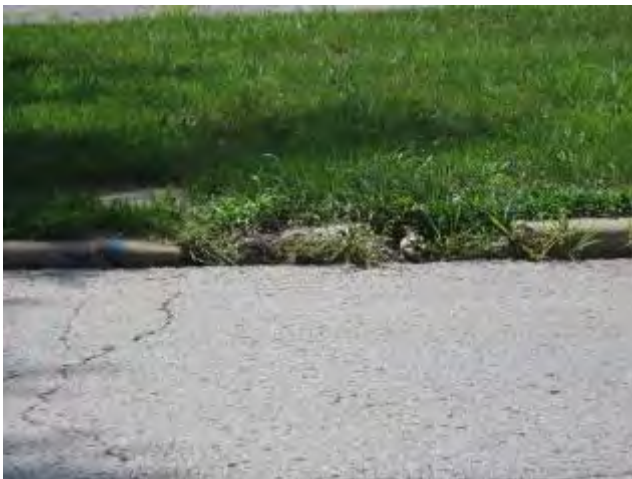
Deteriorated Curbs Along Agnes Avenue
