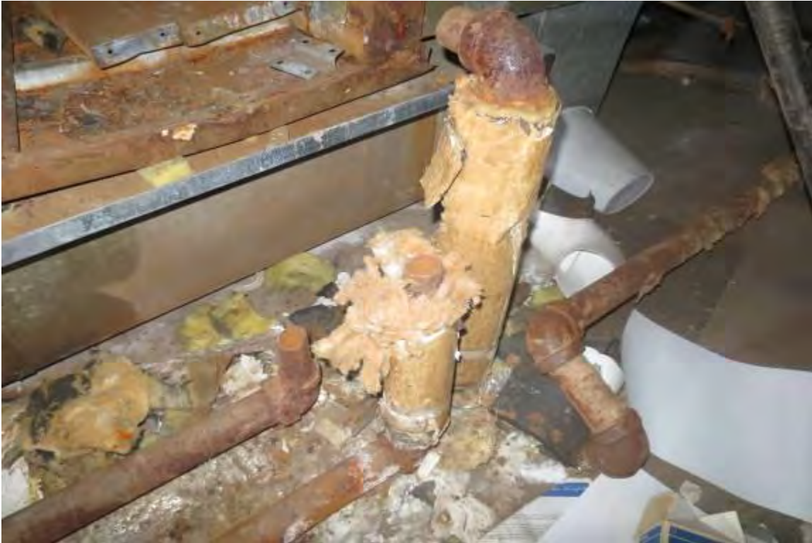
Potential Compromised Pipe Wrapping (ACMs) & Lead-Based Piping – 2801 Swope Parkway
