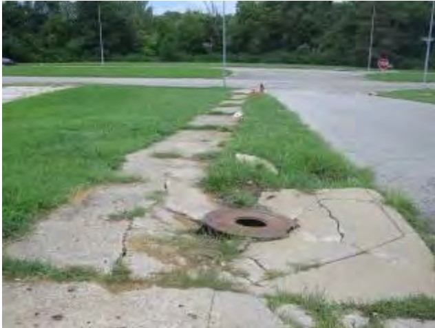
Damaged/Unsafe Sidewalk Along Agnes Avenue
