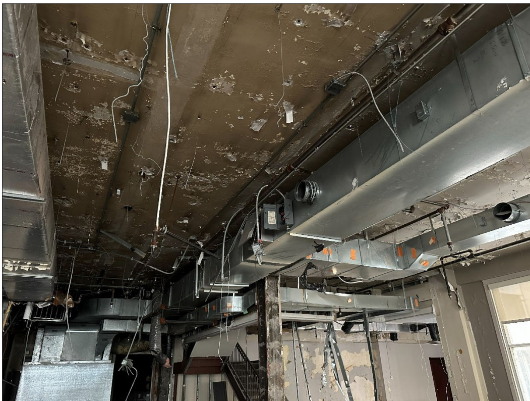
818 Grand Blvd – interior – disconnected, nonfunctioning building systems
