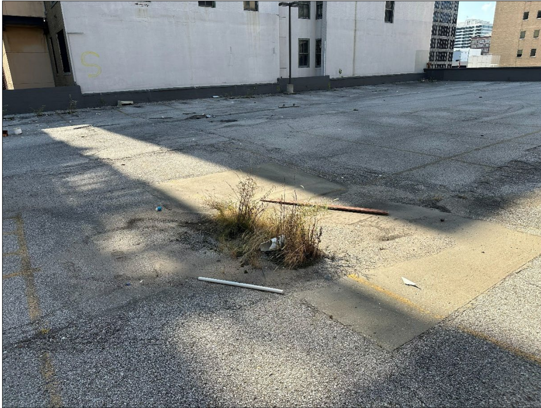
800 Grand Blvd – looking southwest – deterioration of pavement
