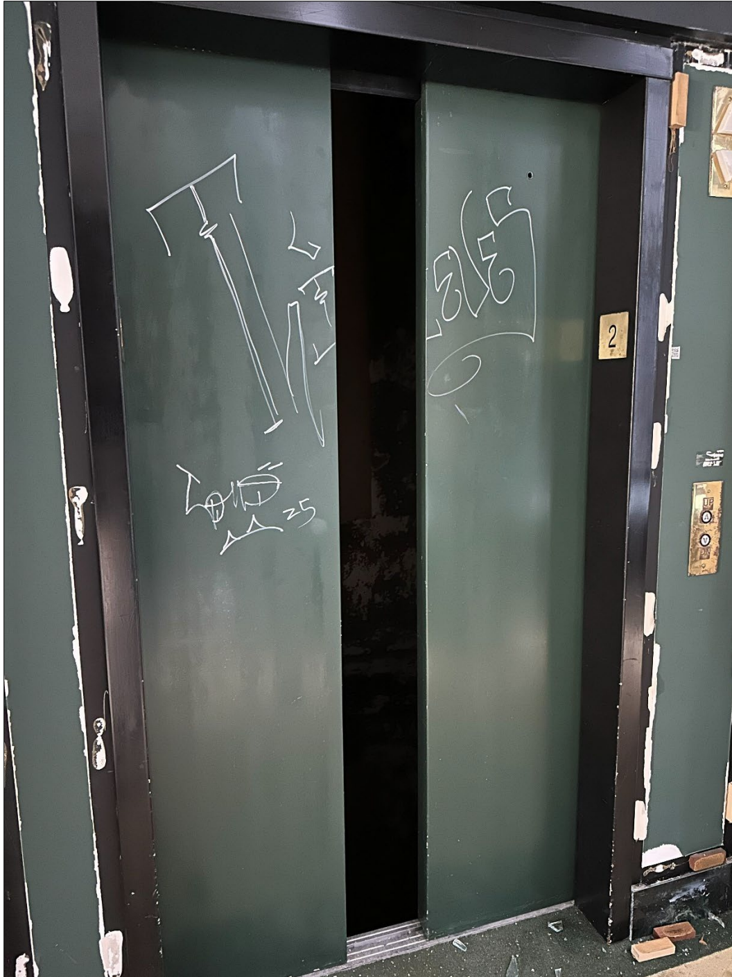
819 Walnut St – interior – open elevator; graffiti
