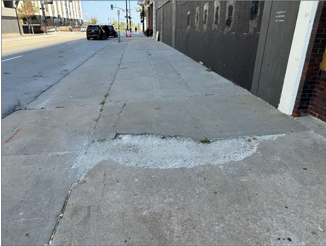
800 Grand Blvd – looking north – uneven sidewalk
