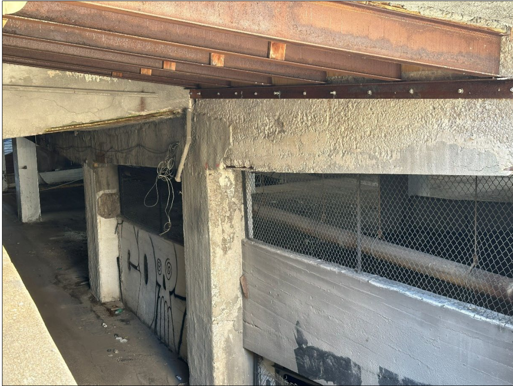
800 Grand Blvd – looking west – spalling concrete; graffiti
