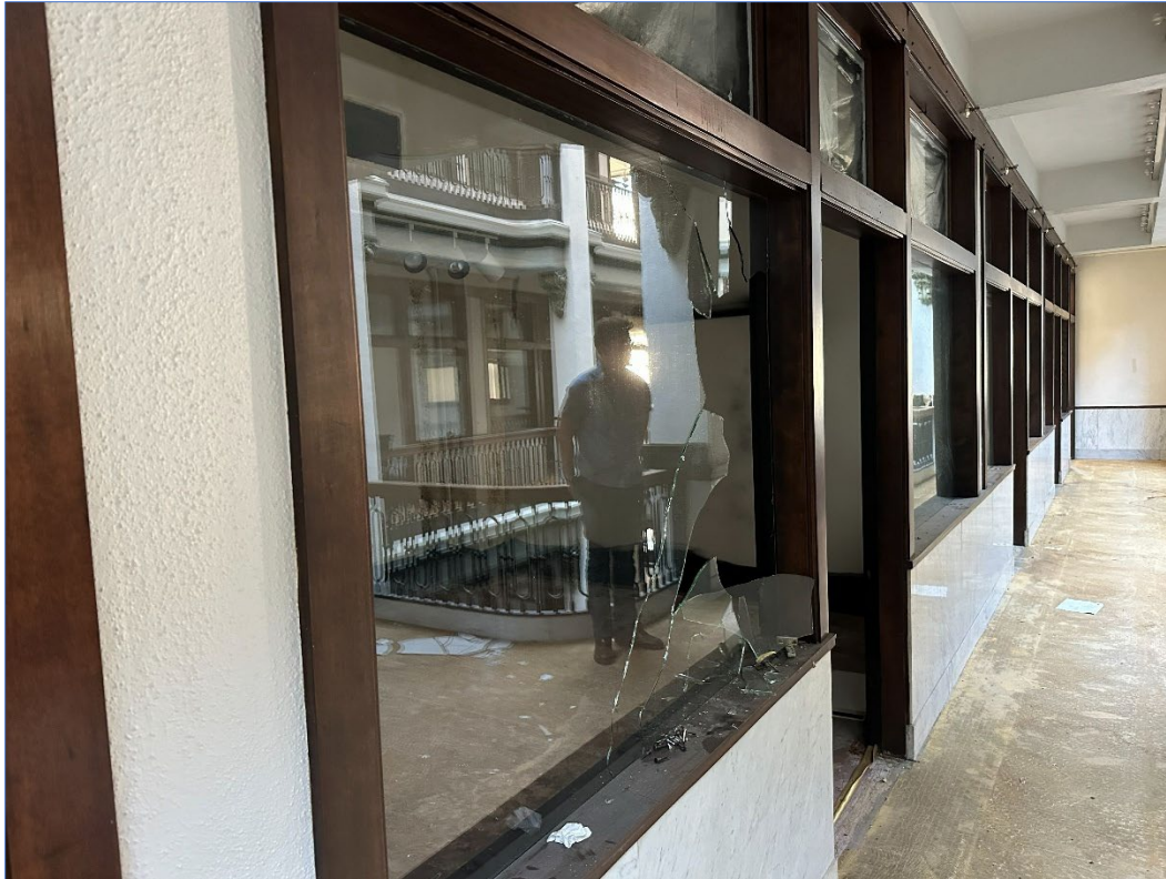
819 Walnut St – interior – broken window (vandalism)
