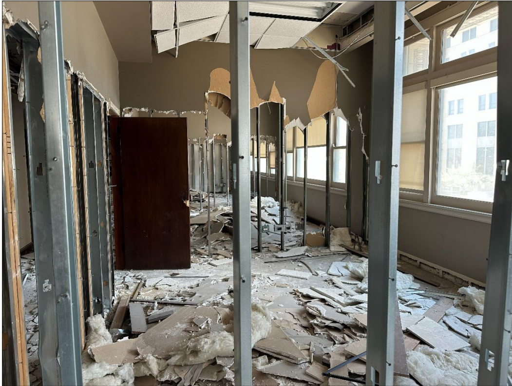
818 Grand Blvd – interior – trash/debris
