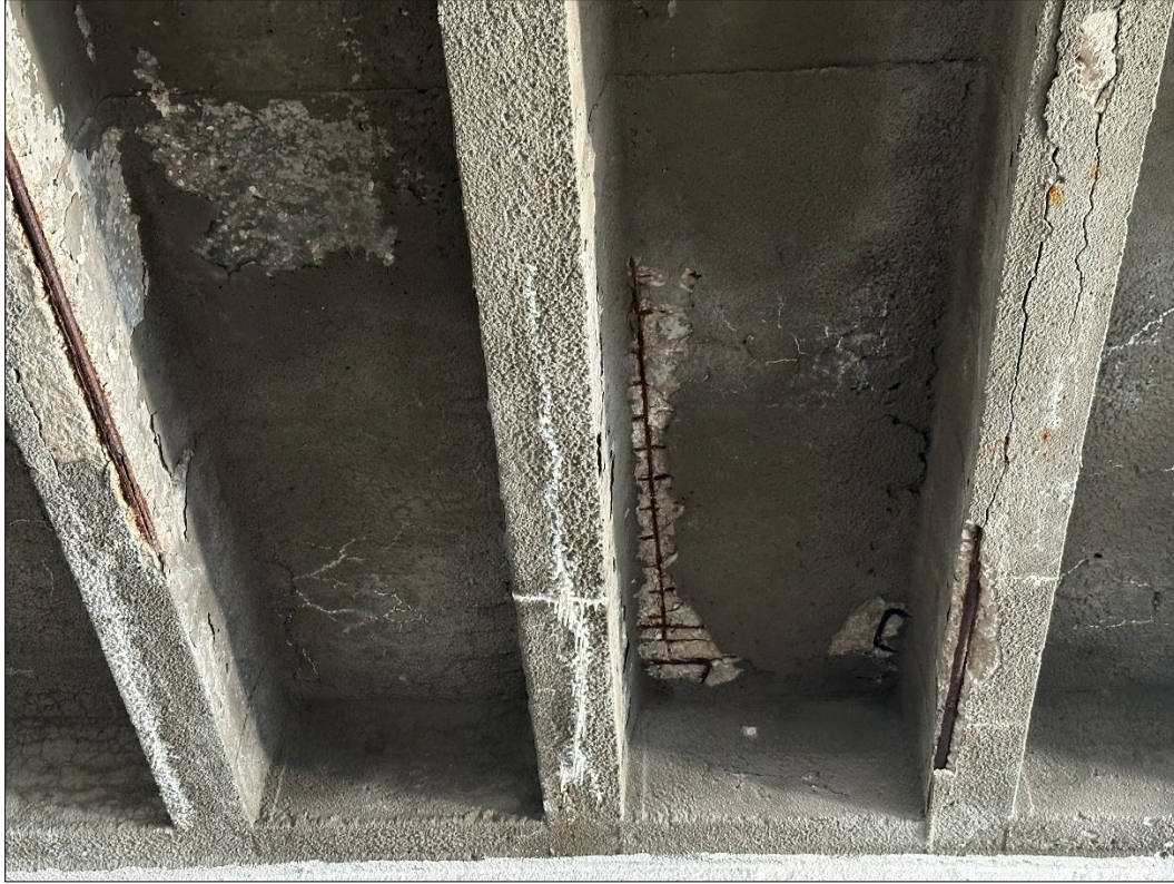
800 Grand Blvd – deterioration of garage structure
