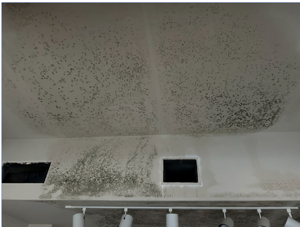
819 Walnut St – interior – mold; failure of finishes
