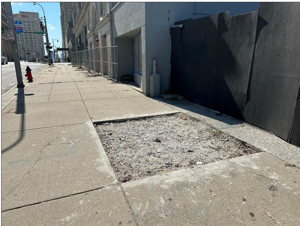
800 Grand Blvd – looking south – uneven sidewalk
