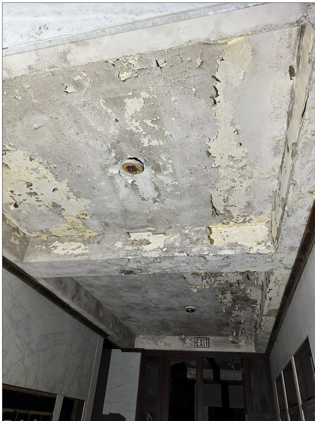
818 Grand Blvd – interior – failure of finishes
