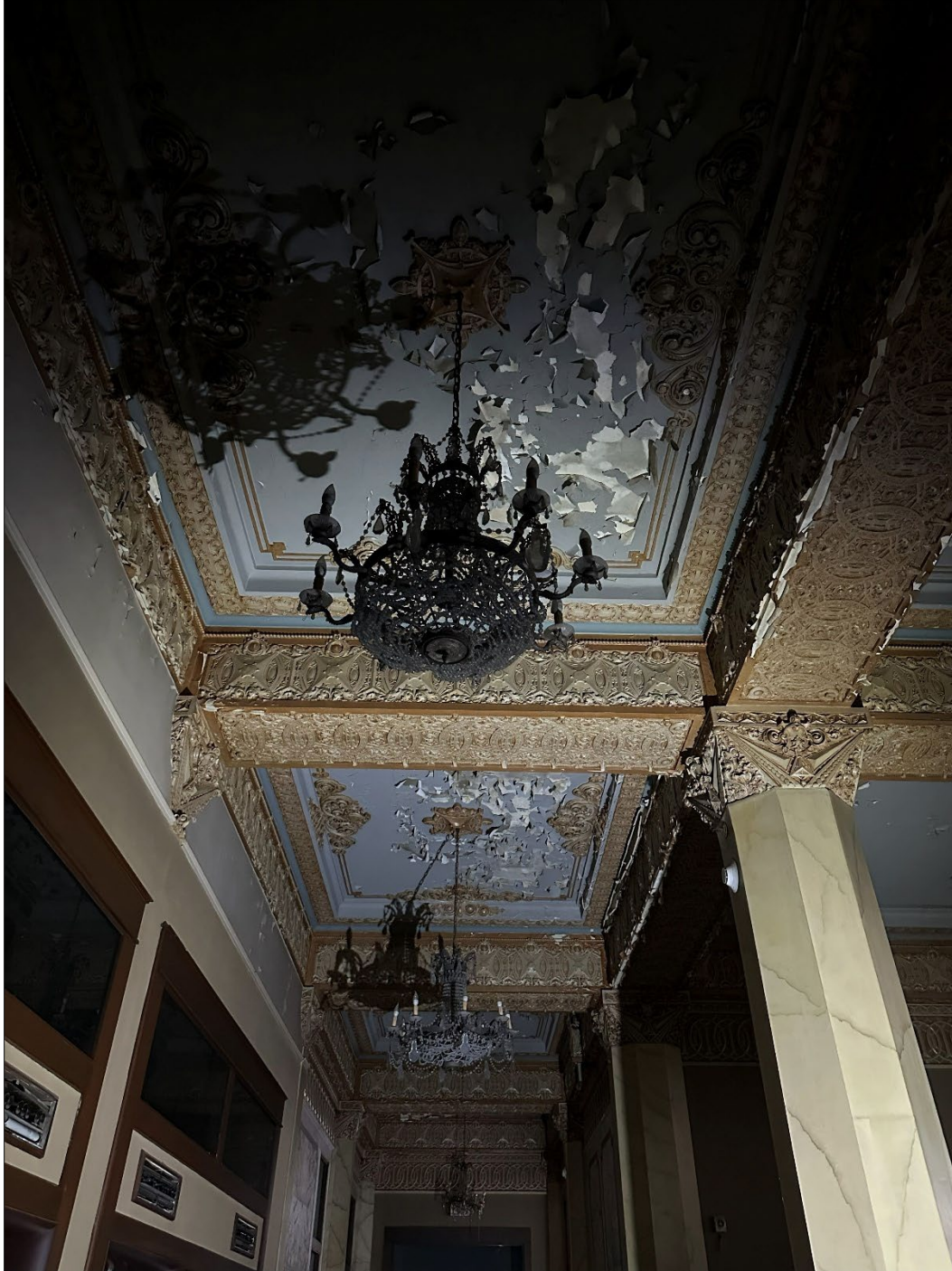
818 Grand Blvd – interior – failure of finishes
