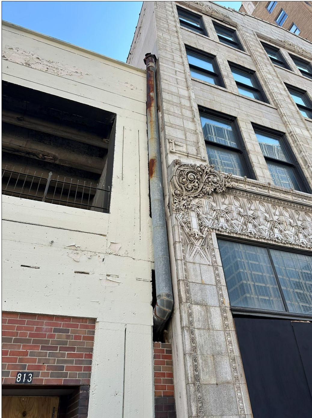
800 Grand Blvd – looking east – rusting mechanical equipment
