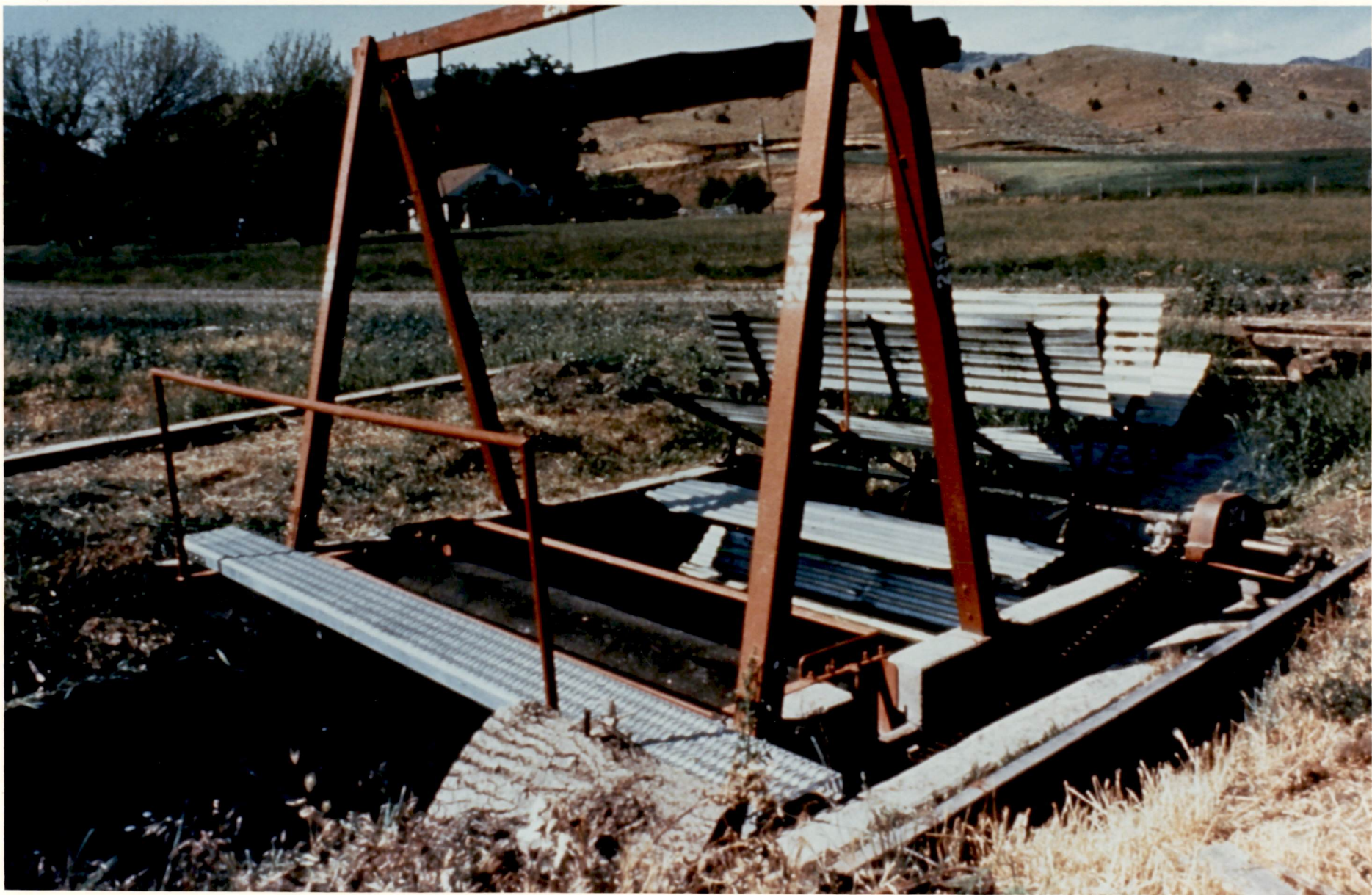
IRRIGATION DIVERSION AND SALMON SCREEN
