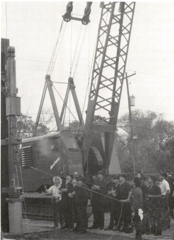
Mr Rick Garcia & Mr Leroy Wesatzke of Pileco, Inc demonstrate the firing of the new Delmag D6-32 Diesel Pile Hammer.
